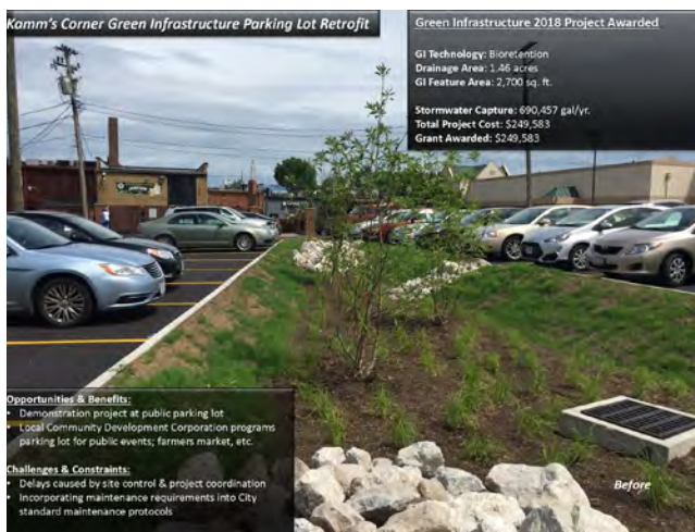
Green infrastructure project for a public parking lot in Kamm's Corners funded by the Northeast Ohio Regional Sewer District
